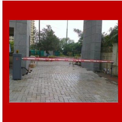
Parking Boom Barrier
